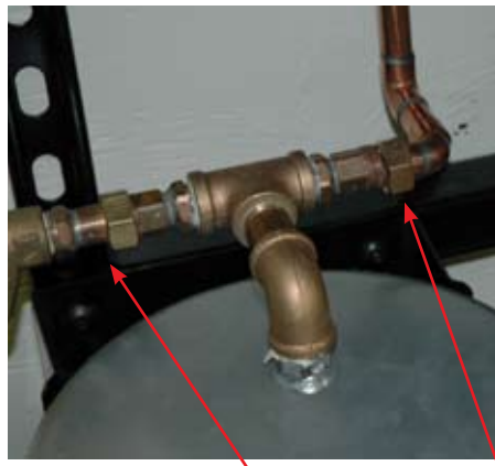
Screw fill valve to union on left side of tank
