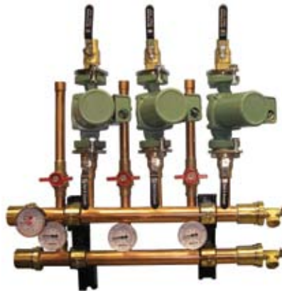
Zone Pumps with Taco 008-F6
