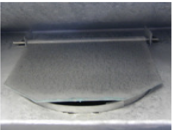
Fig. 11B Improperly closed back draft flapper
